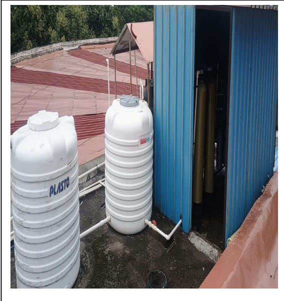
R O Water Filter Project
